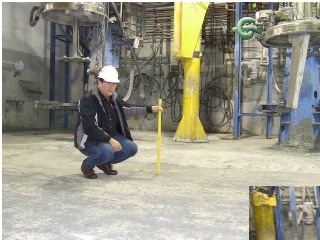
Above – low area causing Unsafe operating condition
