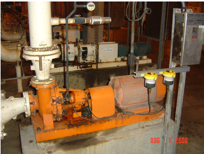
Picture 1: Initial Installation August 1, 2006.
